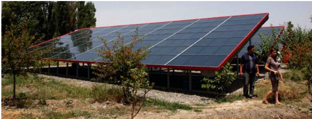
Austrian company Cona is specialised in the field of solar drying. Its air collectors, which can be combined to create large collector fields, are being used here to dry fruit at a facility in Uzbekistan.
